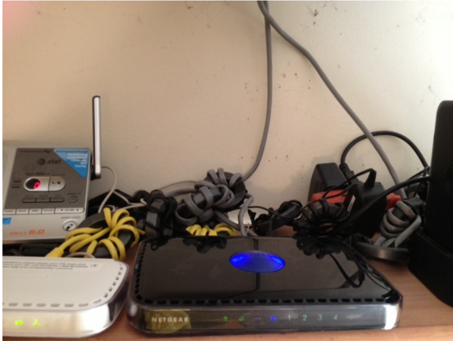
Figure 3 DSL Modem, Router and Network drive (off right in photo)
