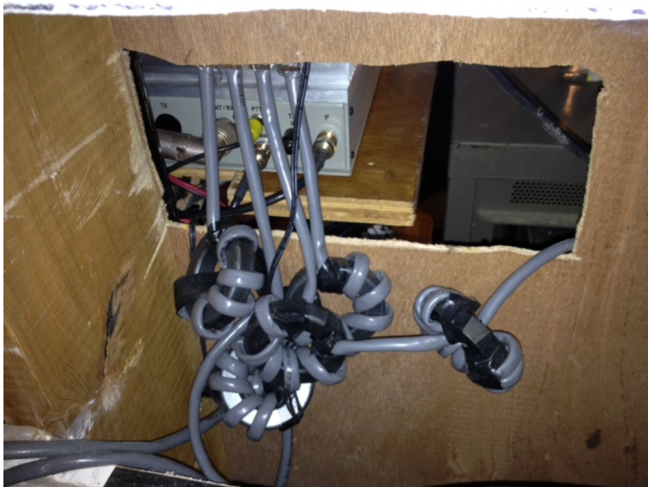
Figure 4 Ethernet Cables at the W5ZN Station Switch
